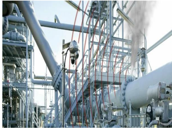
Figure 1: Gas Leakage in industries
